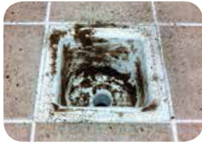
Rusted floor sink
